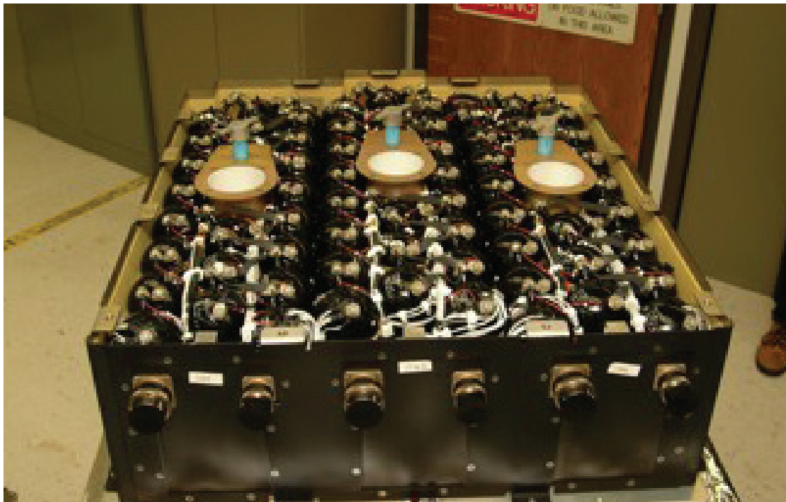
Battery Module Assembly with lid removed, showing the cells and power isolation switches.
