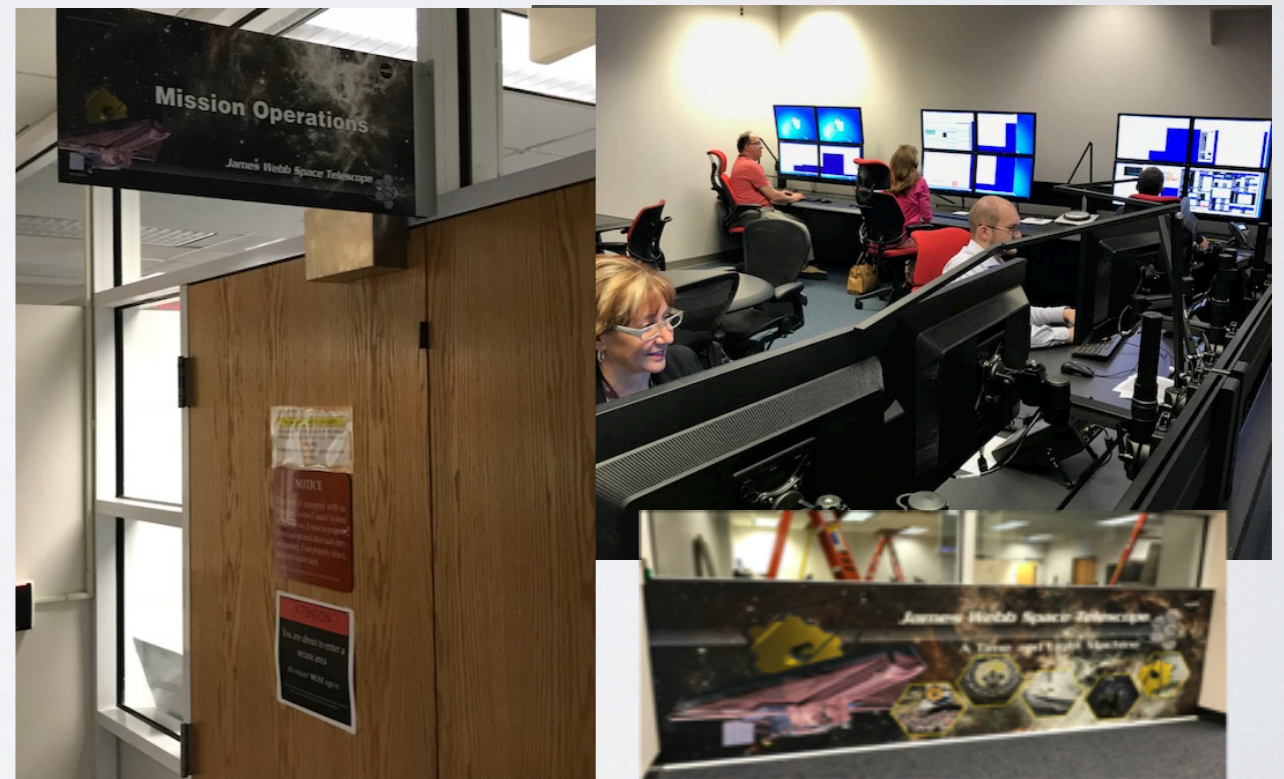
Backup Mission Operation Center (bMOC) in GSFC Building 32
